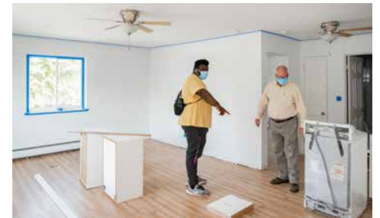
Resident and Shelter For All employee, Justin, discussing with David the final trim out of one of the apartments.
